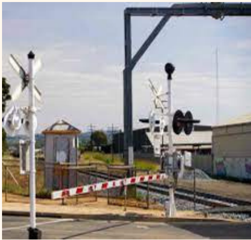
LEVEL-CROSSING GATE CONTROL SYSTEM USING GSM
